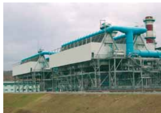
Vacuum Steam Condenser for Combined Cycle; Kulim, Malaysia
