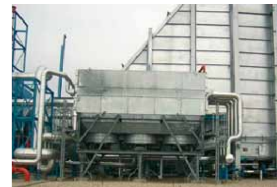
Air Fin Coolers Power Plant, Taiwan
