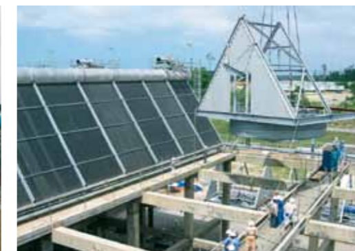
A-frame Air Cooled Condenser Bintulu SMDS, Malaysia
