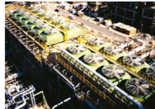
Air Fin Coolers (induced draft) Leuna 2000, Germany
