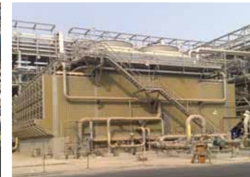
Humidified Aircooler Khursaniyah, K.S.A.
